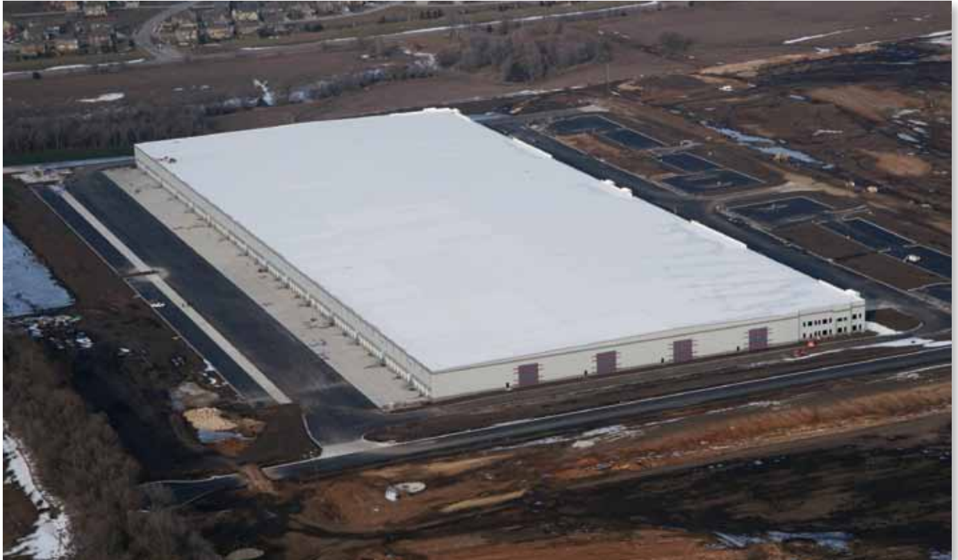
Construction is underway on Building B, an 821,256 sq. foot warehouse in the I-35 Logistics Park. The warehouse is the largest speculative building ever built in the Kansas City area. Sun Life Financial plans to build three bulk warehouses in the 200-acre park.
