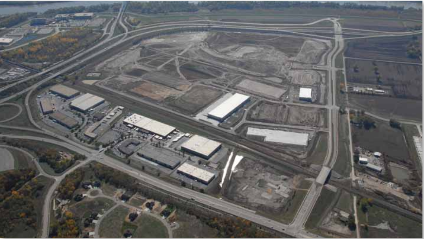
Premium Waters started work on a 160,000 sq. foot, $36 million manufacturing expansion of a private-label bottled water manufacturing and distribution facility at Riverside's Horizons Project.
